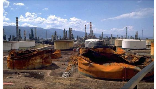
Fig.1 Effects of an earthquake on a process plant.
