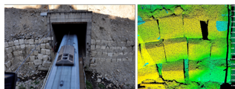
Fig. 2. Lower part of the landslide in proximity of the railway and chromatic representation of block movements (picture by Barbarella).
